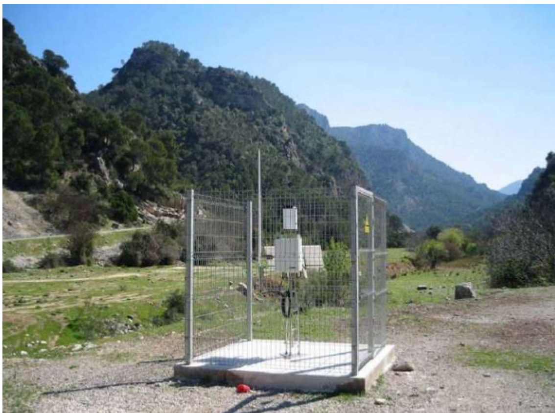
Remote Automatic Rainfall Measuring Station
